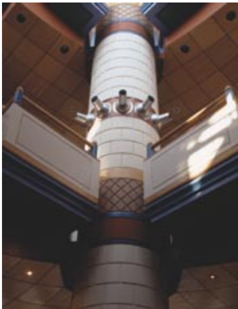
I wanted to put a spotlight into the long-throw air inlet nozzles that recirculated the air down from the 26M-high ceiling. The columns would radiate a diadem of rays of light - proving each one as a 'columna lucis'.
