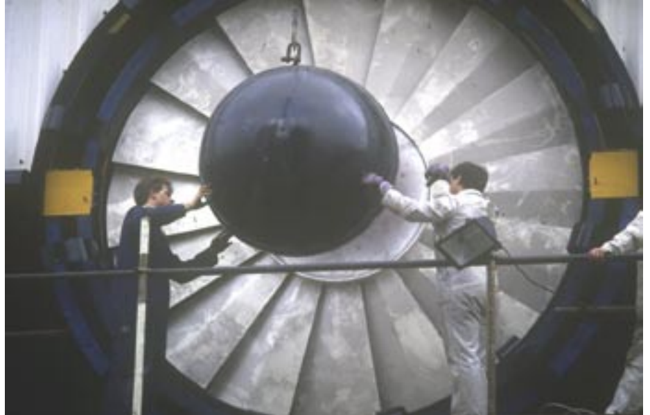
One of the two 3M diam. 'Ventilation Fans' in the Pediment of the Isle of Dogs Pumping Station. It does rotate - although only at a leisurely 16 rpm. What saves it from a merely mechanical triviality is its congruence to both the (Solar) 'Fiery Ember' carried upon the Raft of the Entablature as well as that of the 'Cave between two mountains' from which issues the River of Somatic Time. Needless to say that few will 'read' these latter 'icons'. But that is merely because of the general iconic illiteracy - an 'Architectural' state that these 44 Lectures aims to relieve!
